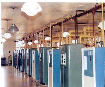
Disinfectant Metered by Chlorinators.
