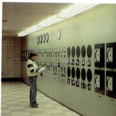
Master Control Panel.
