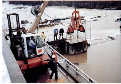
Operators Clean Intake Bar Screens.
