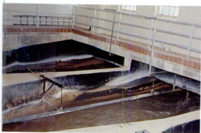
Chemicals and Raw Water Being Mixed.
