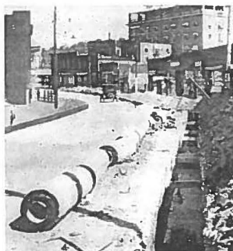
ADSCO Casing installed in Excelsior Springs, Mo.
