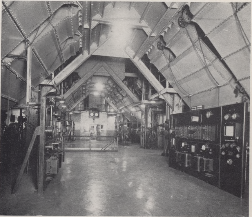
Fig. 11—Boiler Room, Beacon Street Heating Plant
