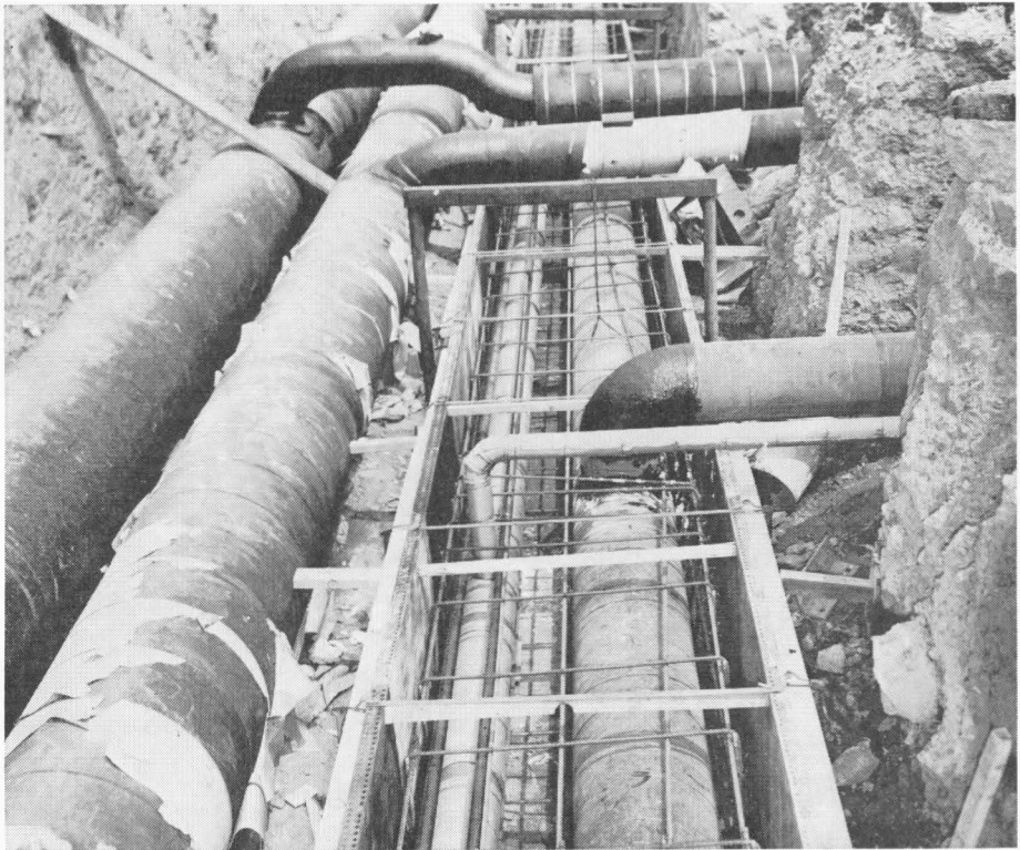
FIG. 6—Underground piping system: left to right; 30-in. chilled-water supply, 30-in. chilled-water return, 8-in. condensate return, and 12-in. steam supply. Take-off lines on right are service connections for Sears Department Store and Shopping Mall. Also shown are forms for encasing steam and condensate lines in concrete envelope.
