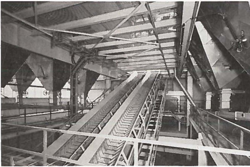
Conveyor system in Spittelau carries garbage from storage to feed the dual boilers. The two belts are interconnected to permit changeover in the event of breakdown.
