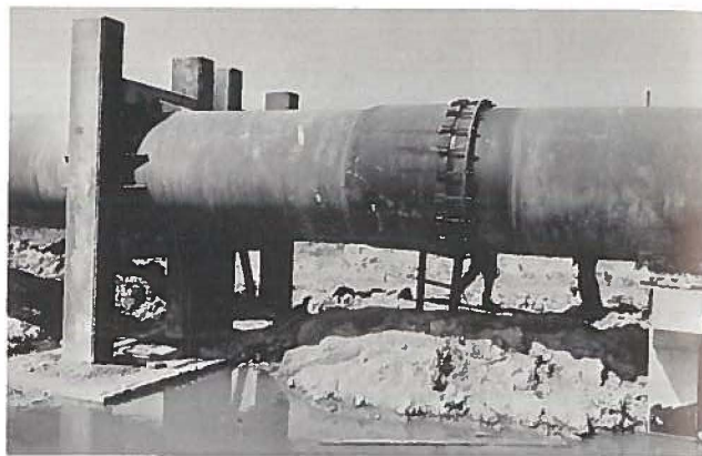
Fig. 9—Leningrad: supply and return mains above ground, with expansion joint.
