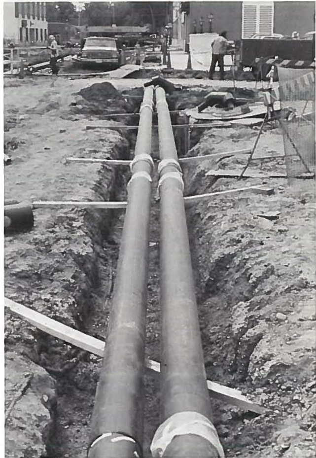
The pipe was welded and hydrostatically tested before being lowered into the ground.
