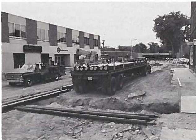
Pipe was delivered for the district heating system, which was the first utility to be installed in the redevelopment.
