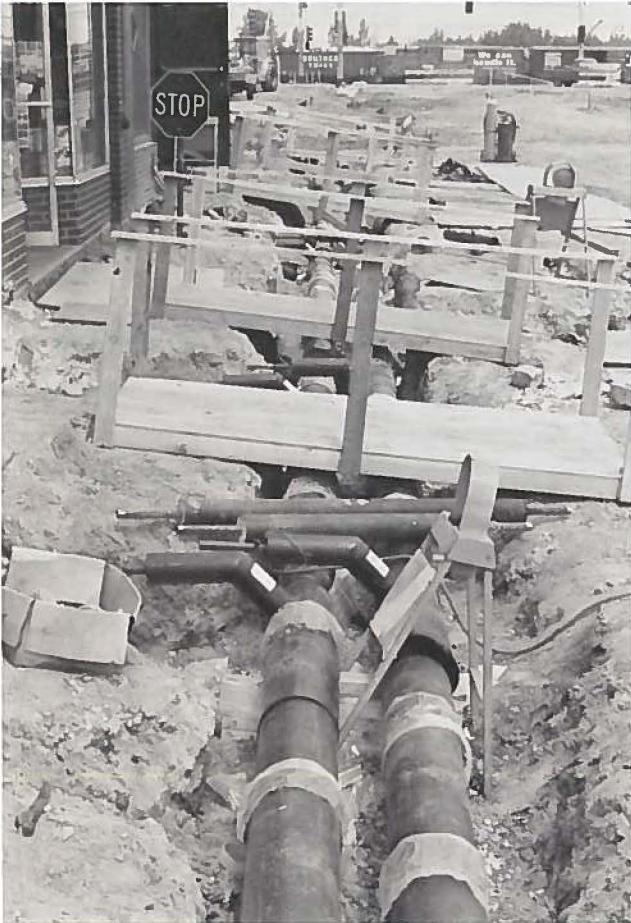
The piping was fitted to make the connections to the individual buildings.
