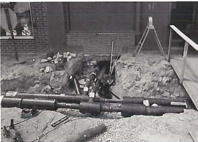
A connection is made to one of the many businesses on the new district heating system.
