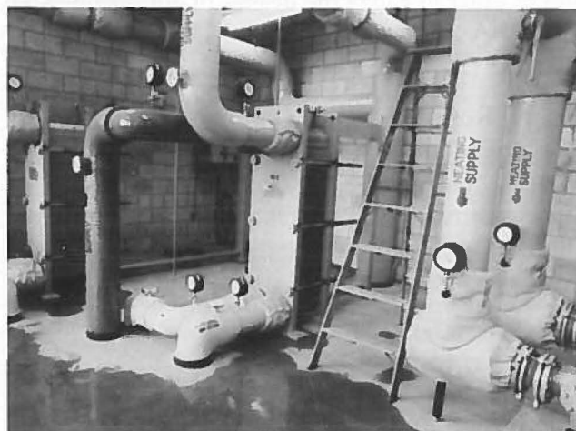
Figure 6 Heat Exchangers and Pumping Station
