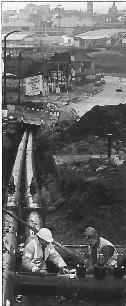
Workers inspect a bend in the district heating system piping in Sheffield.
