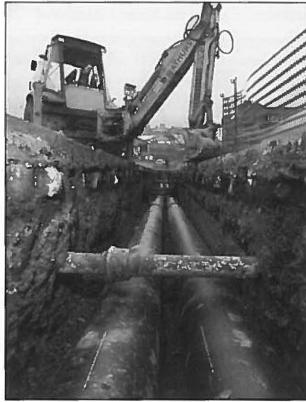
The piping was strategically designed to negotiate the utility interferences often found beneath the streets.
