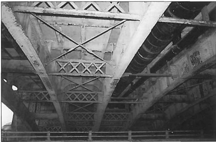
Steam and condensate piping can be seen in the right half of this photo taken from under the Longfellow Bridge.
