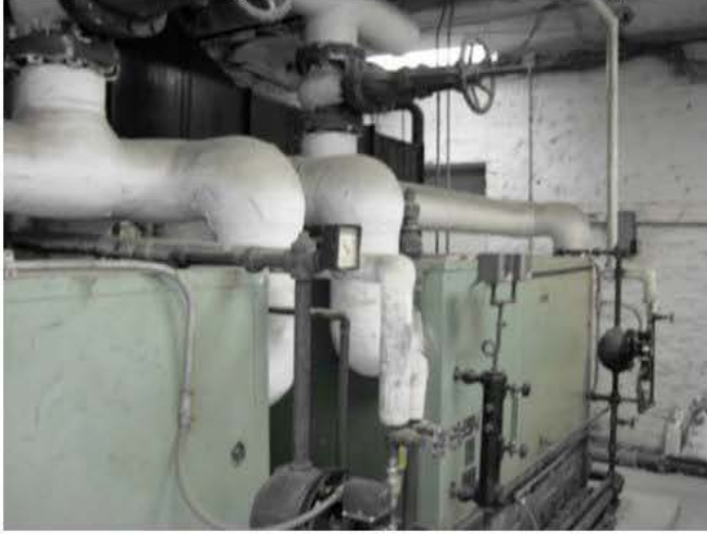
Columbia County Courthouse Boiler Room, Basement
