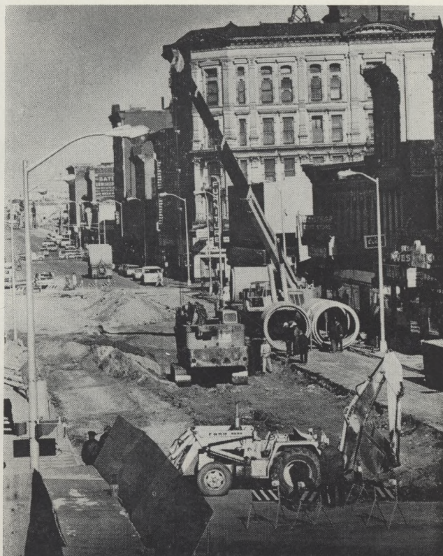
FIG. 1 — Installing new steam mains in lower downtown Skyline Urban Renewal District. All old buildings in photo will be razed.
