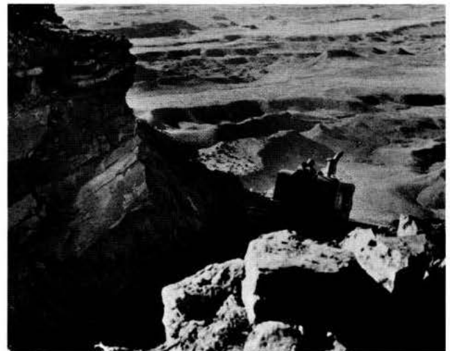
A bulldozer cuts a trench for the Hunters Canyon line of Western Slope Gas Company near Grand Junction in the fall of 1966. Difference in the highest and lowest wells on this system was 1,200 feet.
