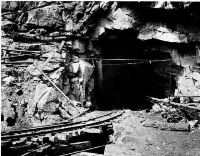
Diversion tunnel carrying water from the Colorado River to the Shoshone Hydroelectric Plant is 2½ miles long and bores straight through the granite wall of the canyon.
