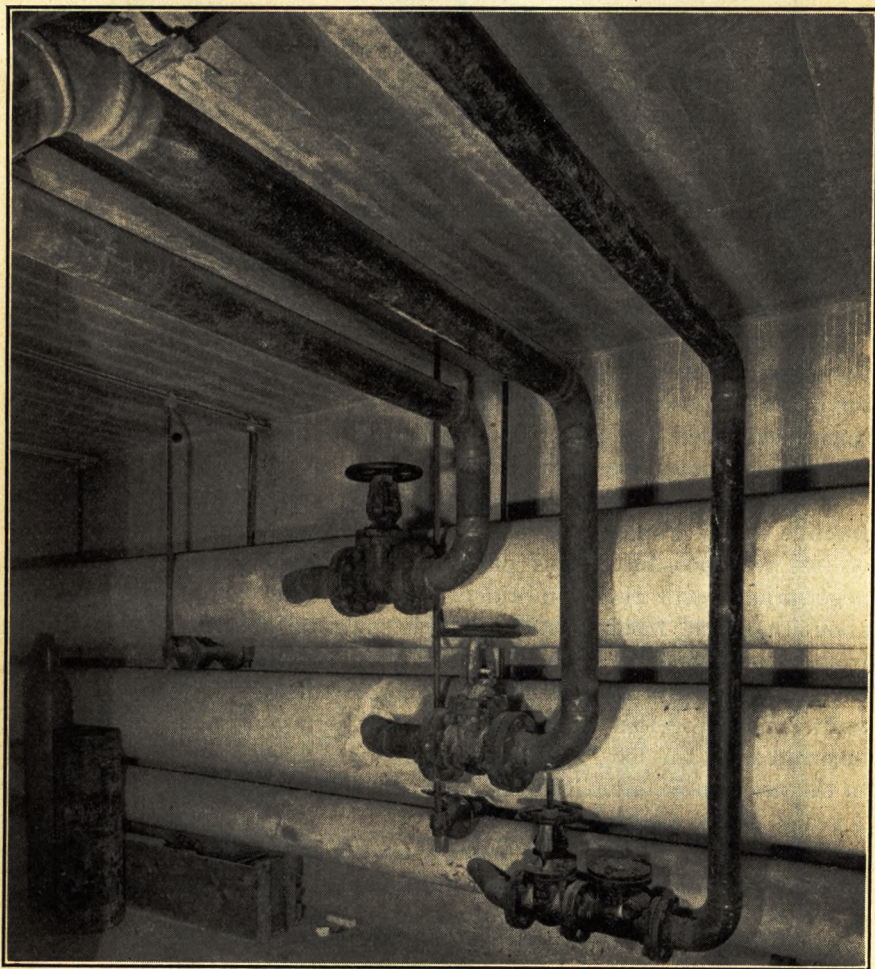
Steam and return connections to Dunster House.
