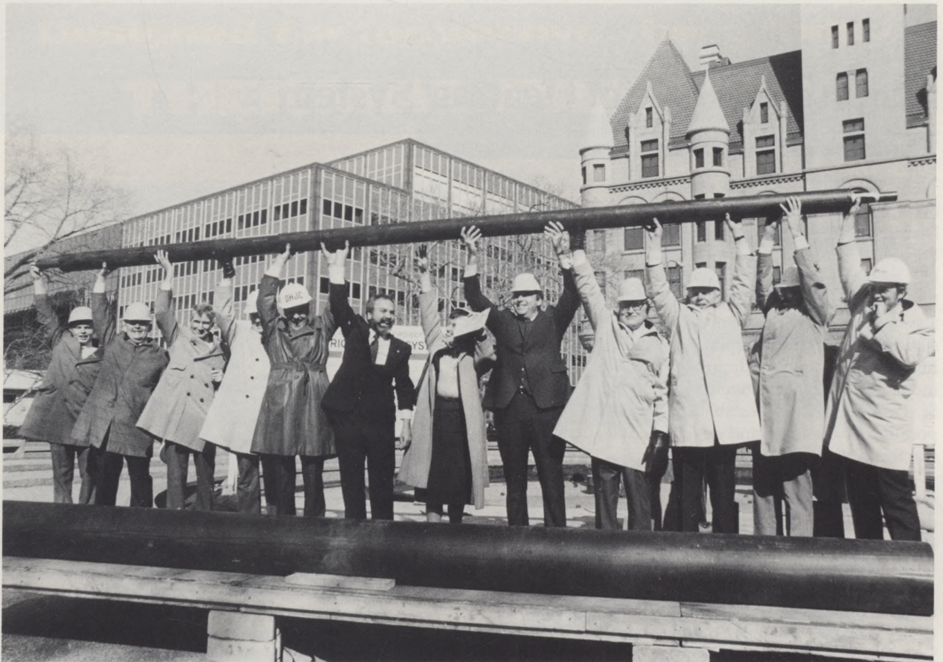
The laying of the first pipe was the highlight of the days events. Participants in the event were, from left to right: Dr. Michael Karnitz, Oak Ridge National Laboratory; Norman Taylor, International District Heating Association; C.S. McCrossan, C.S. McCrossan Construction Co.; John Mullen, First National Bank St. Paul; Hans Nyman, District Heating Development Co.; George Latimer, Mayor of St. Paul; Barbara Lukermann, DHDC Board member; Stuard Sloame, U.S. Department of Housing and Urban Development; Phil Fuller, HDR; Cliff Olson, DHDC Board member; Kent Shamblin, DHDC Board member; Cliff Bowers, Metcalf & Eddy.
