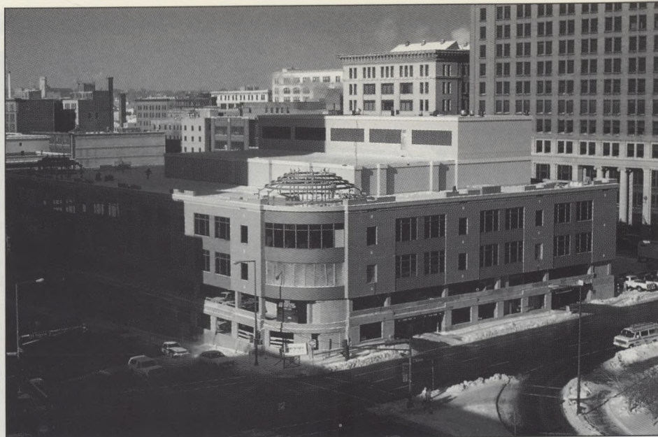
Minnesota TeleCenter, future home of KTCA-TV Ch. 2 and KTCI-TV Ch. 17, under construction in downtown St. Paul. Courtesy of KTCA-TV
