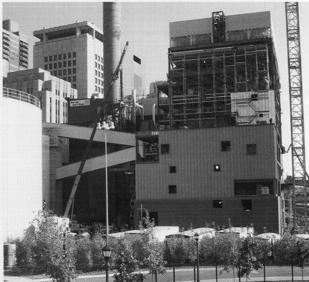
Completion of the combined heat and power plant (above), fueled by urban wood residuals, is scheduled for this winter. The existing boilers will be used as needed during peak demand periods.
