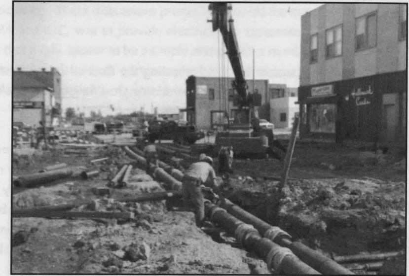
New heat lines, ready for installation
