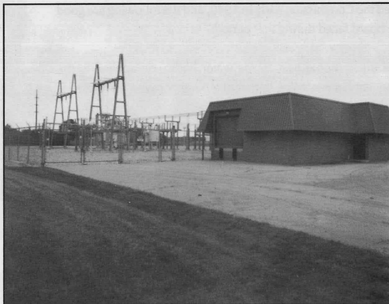
South Sub-Station, 19th Av. SW and 9th St.
