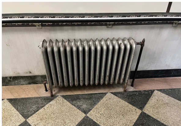
Photo 3 - Typical Steam Radiator - Corridor
