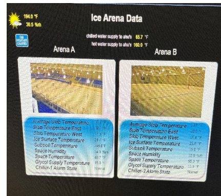
Photo 9 - Ice Rink BMS Screen
