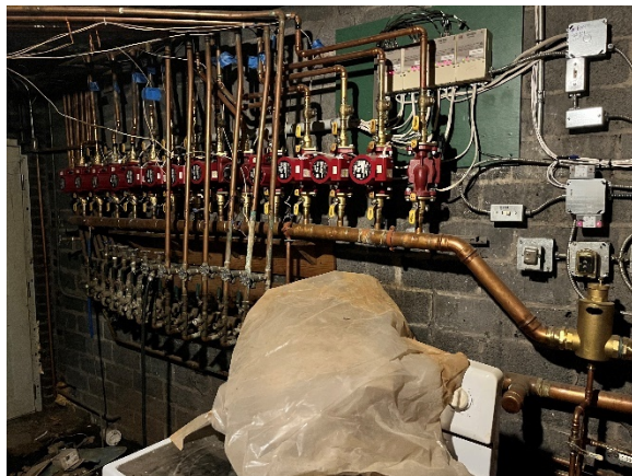
Photo 21 - Jefferson St. Apartments - HW Circulator Zone Control
