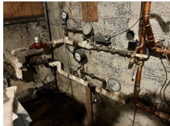
Photo 22 - Jefferson St. Apartments - District Heat Supply & Return Pipes
