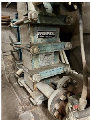
Photo 5 - Heritage Park - District Heat Plate & Frame HX
