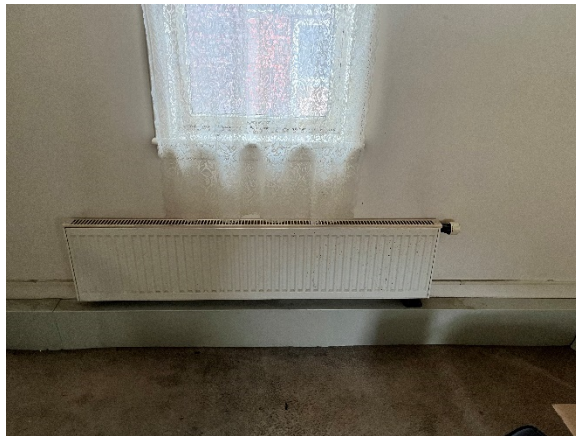
Photo 11 - Covenant Manor Panel Radiator
