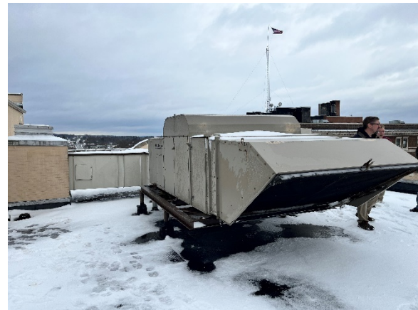
Photo 12 - Rooftop Air Handler
