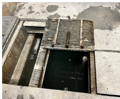
Photo 8 - Ice Rink - Ice Melt Pit
