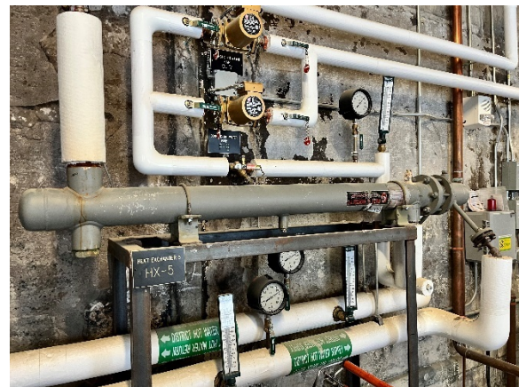
Photo 20 - Comedy Center - DHW HX
