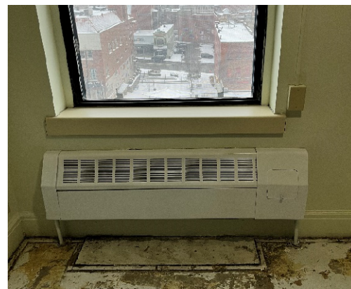
Photo 4 - Typical Finned-Tube Unit - East Apartment
