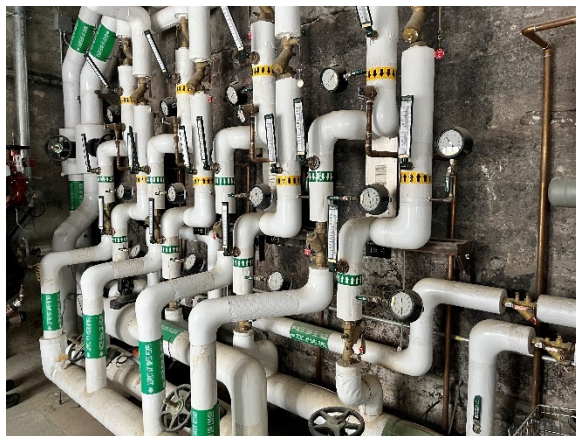
Photo 19 - Comedy Center - Space Heating HX's
