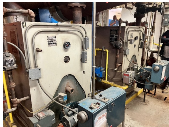
Photo 6 - Heritage Park - Backup Boilers
