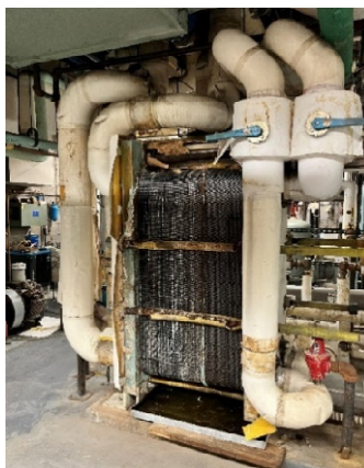
Photo 2 - District Heat to Bldg HW Heat Exchanger
