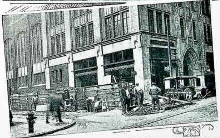
New steam main construction: Top, At Main Street East, looking south on Stone Street; Center, On Gibbs Street, at Main Street East, near the Eastman Theatre, and, Bottom, On North Street, in front of Baptist Temple. This line also serves the new Rochester Savings Bank, just across from the Temple Building.
