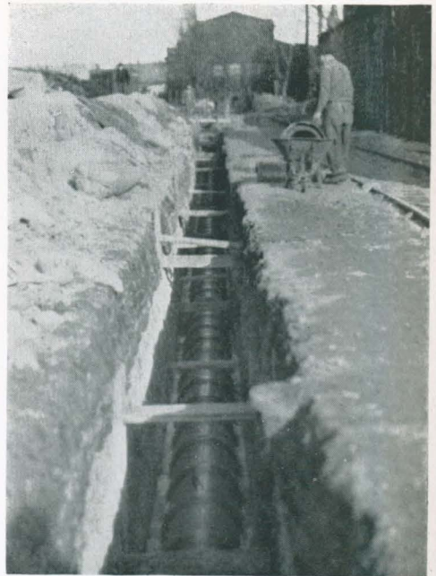
Ric-wil Dry-packT Conduit in Trench alongside active railroad siding. Frozen ground aided construction by holding up trench thru loose, shifty sandy loam.
