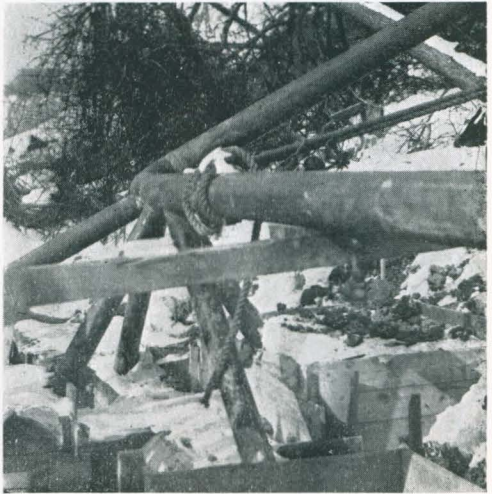
Main Anchor at foot of hill. 4" pipes, welded on after main was run, anchored in concrete blocks.
