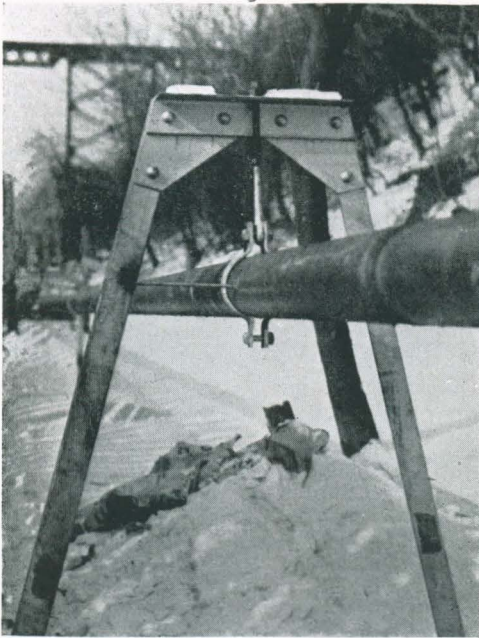
Typical A Frame Support—holding 6" High pressure main before insulating.
