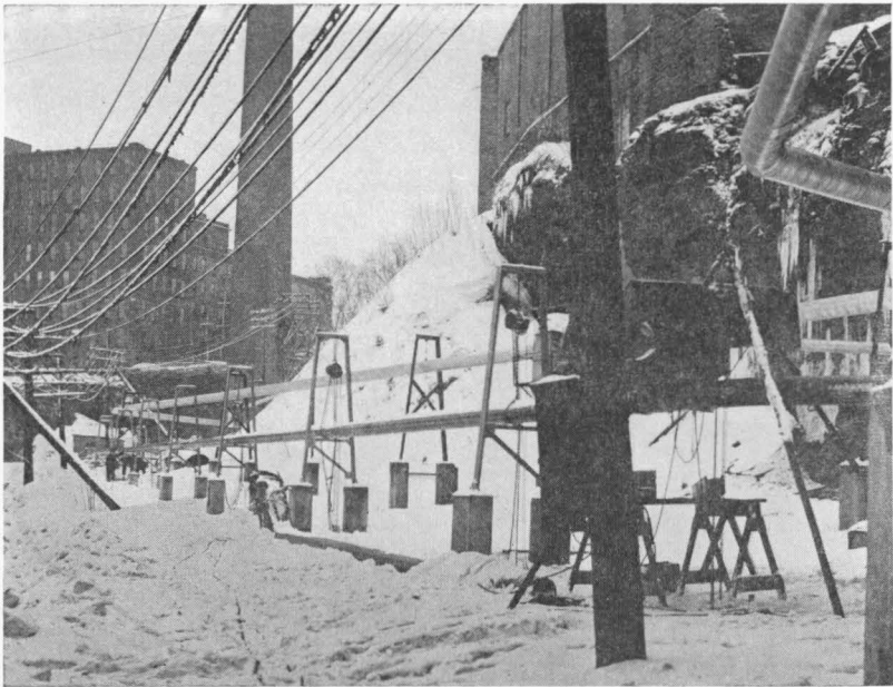
FIG. 2.—For 812 Feet the Line Suspended from Steel Supports Passes Through Part of the River Gorge.
