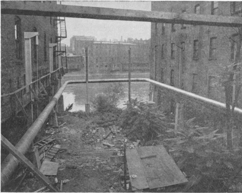
FIG. 7.—The Expansion Loop Takes Care of 5 to 6 Foot Changes in 1000-foot Straight Run of Pipe Located in Raceway.
