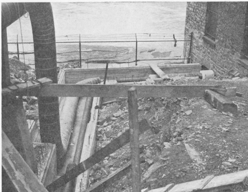
FIG. 1.—Insulated 10-Inch High-Pressure Steam Transmission Line Emerges from Station No. 3, of Rochester Gas and Electric Corporation, which is located on the Genesee River.
