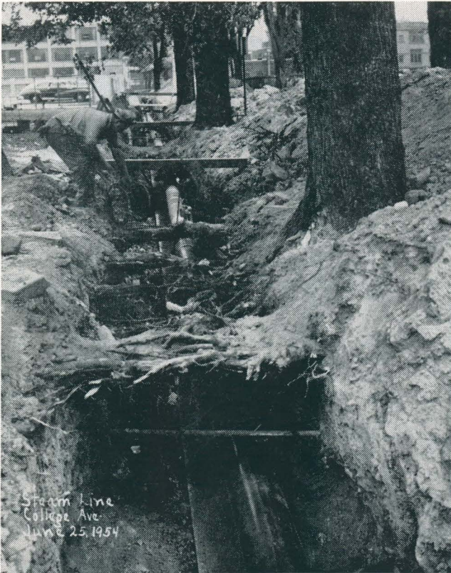
Steam Line—College Ave., June 25, 1954
