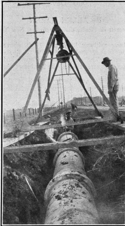
At the End of the Pipe in Place. The Horse Moves Along on Rollers to Handle the Next Section
